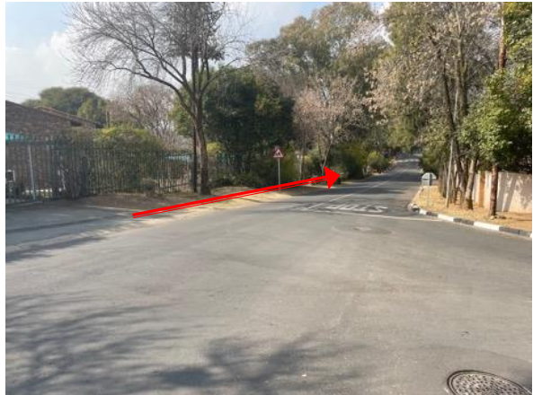
Figure 9 – Alignment down garden road (corner of valley and Garden). Existing sewer manhole in the right corner of the picture.
