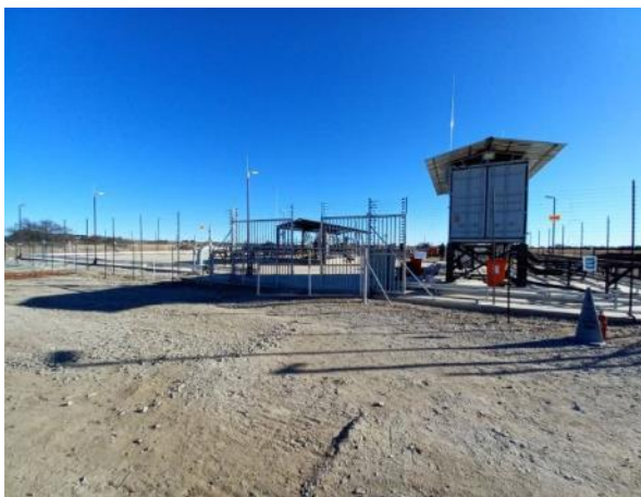
Figure 11: Centralised Compressor station.
