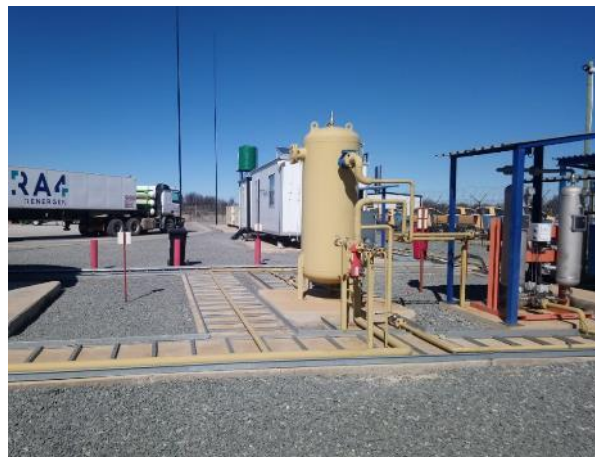
Figure 18: HDR1 Production well and associated facility.
